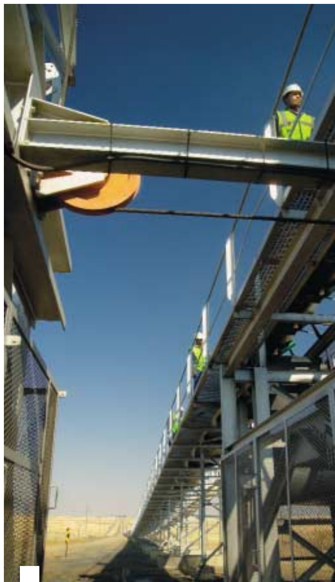
The new Mooikraal mine near Sasolburg in South Africa was brought into operation, including the new conveyor system for supplying utility coal to our Sasolburg petrochemical plant.
