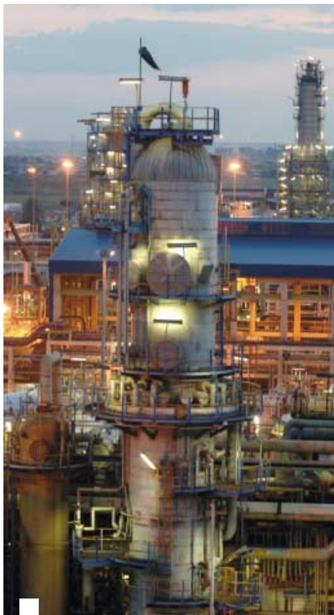
The uprated vinyl chloride monomer (VCM) plant at Sasolburg with a view of the new 220 000 tpa low-density polyethylene (LDPE) Project Turbo plant and the older, recently uprated 150 000 tons per annum linear low-density polyethylene (LLDPE) plant behind it.
