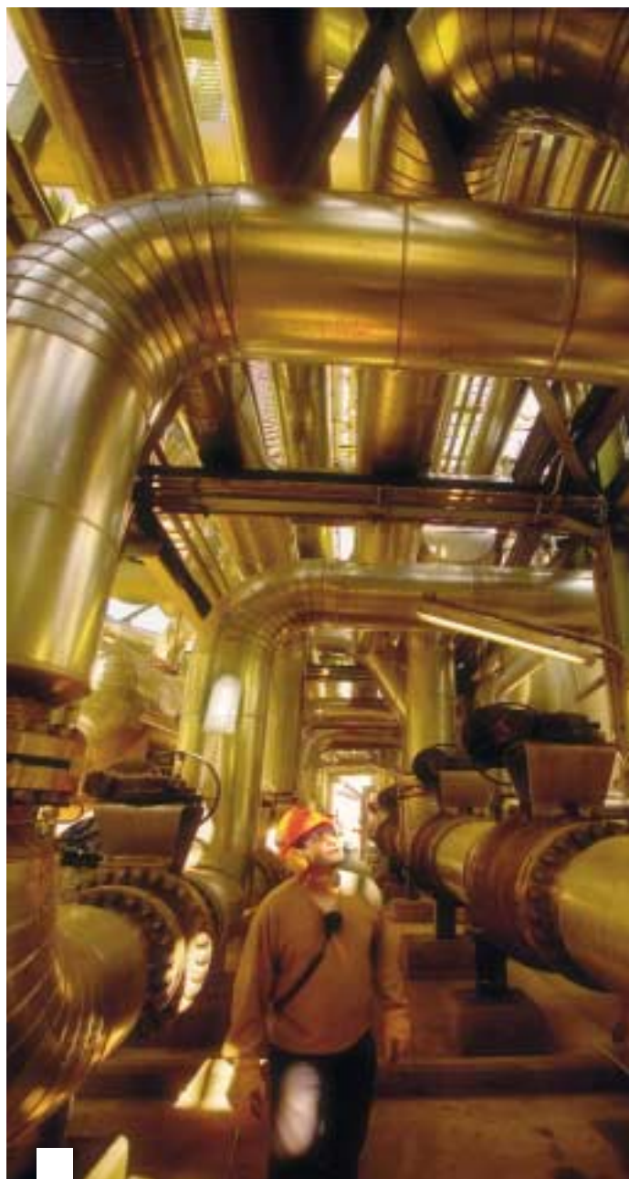
Work in progress for the Project Turbo fuel-optimisation and polymer-expansion project at Secunda, our biggest South African project since commissioning our original Secunda facilities in the 1980s.
