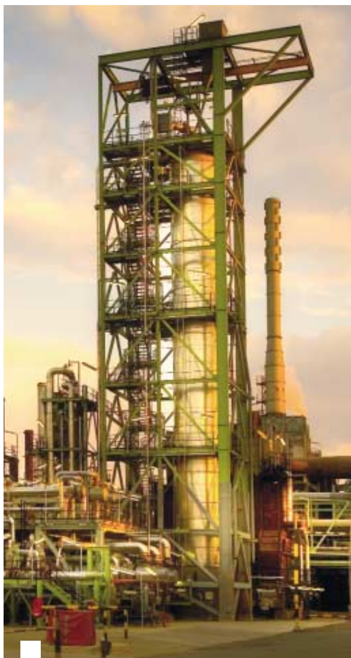
The diesel unifier that was installed during the Natref clean-fuels project at Sasolburg during 2005. Since January 2006, Natref has been producing diesel with a reduced sulphur content of 500 ppm.
